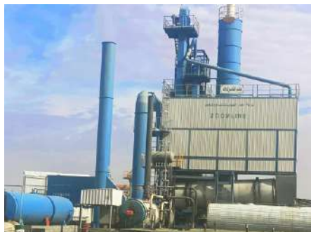
ZAP-S200 Asphalt Plant in Saudi Arabia
