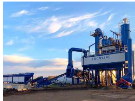
ZAP-S120 Asphalt Plant In Kazakhstan
