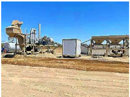
ZAP-C40 Asphalt Plant in Kazakhstan
